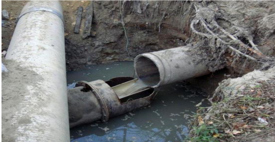
Figure 1. The sewerage collector from the “Propeller area” 1
